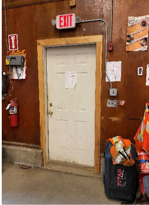
Photo 5: Updated emergency signage/lighting
