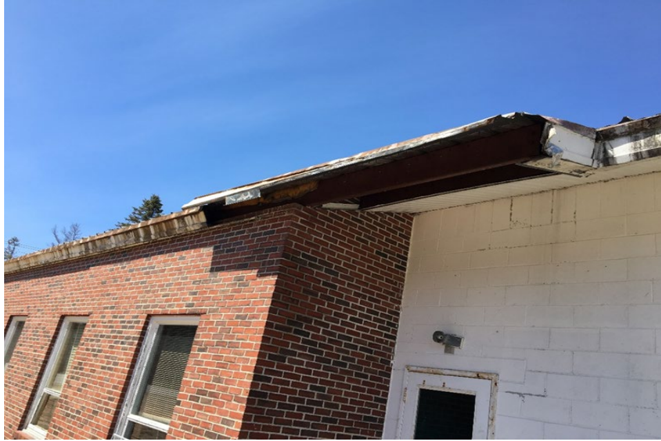
Photo-3: Close-up view of the holes in the trim and soffit where pigeons and animals gain access to the interior of the building.
