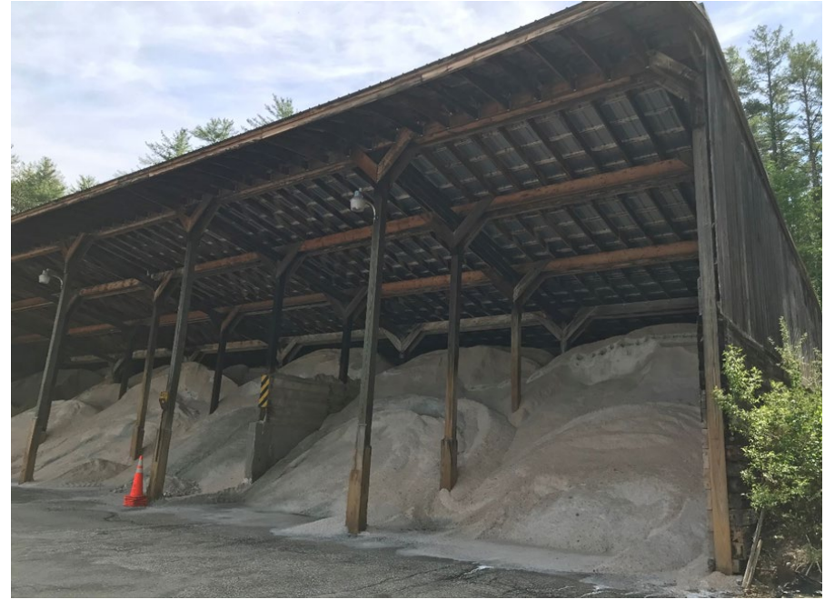
Photo 6: Warner (526) – Salt Shed Inadequate Capacity
