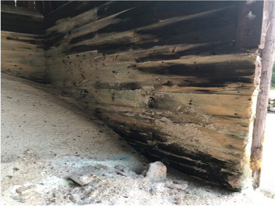
Photo 5: Belmont (314) – Deteriorated Wall Condition
