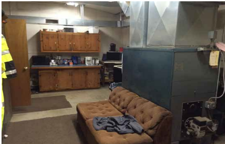
Photo 1: Furnace w/out fire separation; crew rest area in public space
