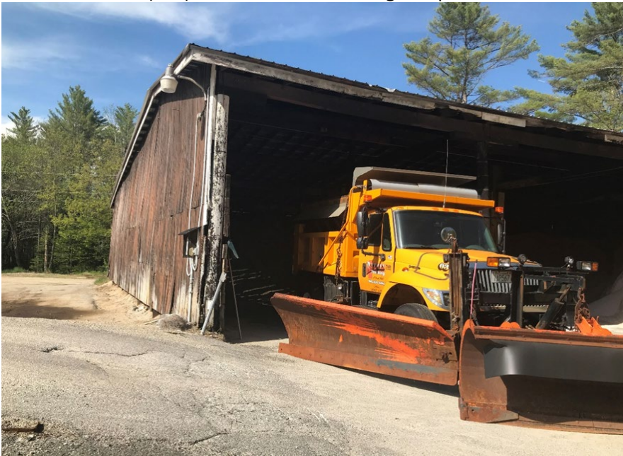
Photo 3: Lempster (215) – Salt Shed Deteriorated Condition
