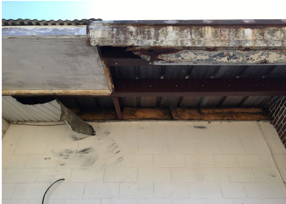
Photo-6: Closeup view of additional holes in roof trim and soffit.
