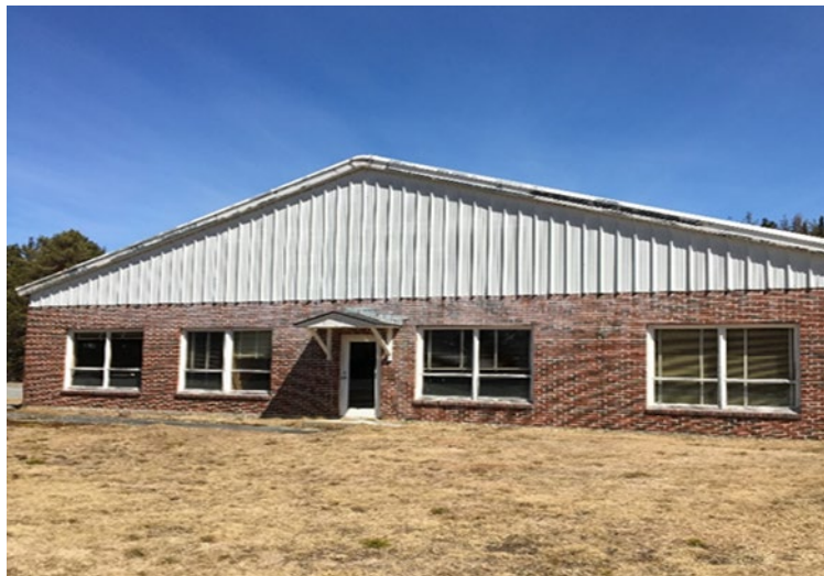
Photo-4: View of the front of the building. Note single pane, outdated windows and deteriorated siding and rotten trim.
